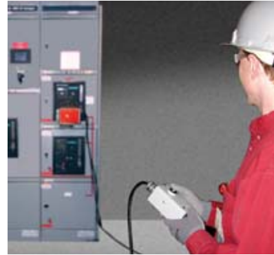
Remote Racking Device
