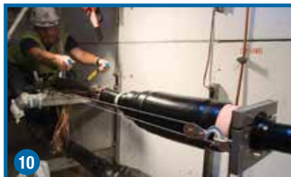
10 Reposition the assembly tool and pull the TCJ joint housing into the final position on the cable.
