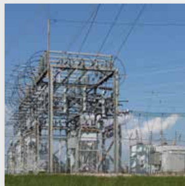
Transmission and Distribution
