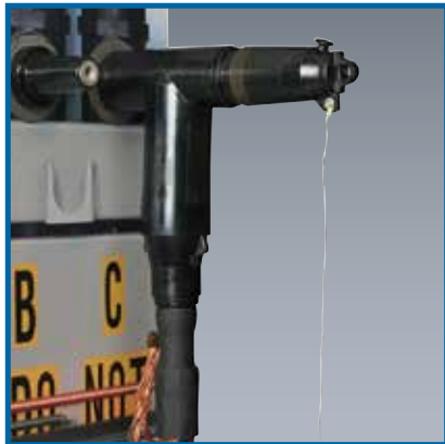
ComboT CETP installed.
