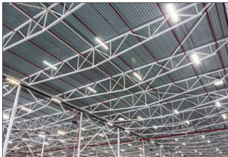
EPCO 4-foot LED Vapor Tight Luminaires powered by our 277 Volt Illumination Control Fixture Whips.
