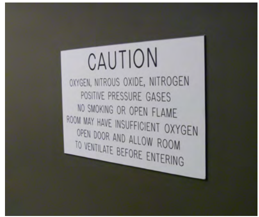
Figure 19. Equipment Room Wall Plate.
